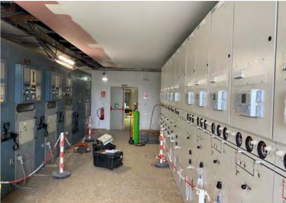
New bays in the Langreo substation
